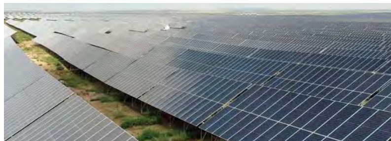
The Large-scale Photovoltaic Composite Project in Yanchi, Ningxia
