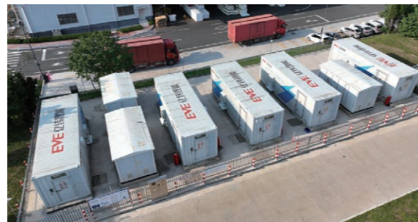
Hisense Huangdao Information Industrial Park Energy Storage Equipment
