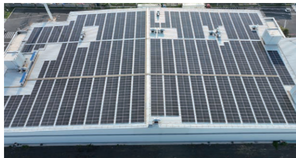
Factory Roofing with Photovoltaics
